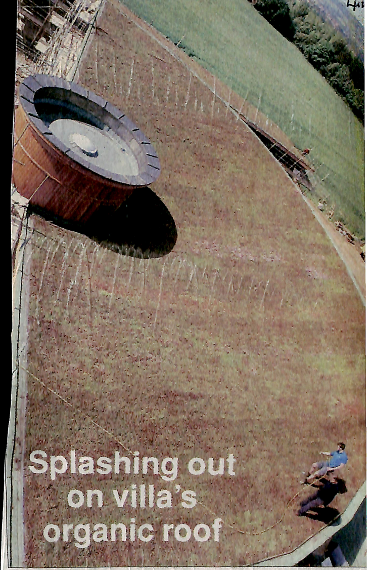
Brading Roman Villa site manager Nigel Meaden prepares to new sedum roof covering. Picture by CHRIS THWAITES 0604-c14
