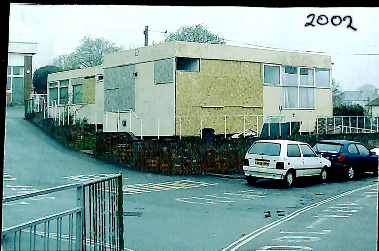
Work has started on conversion of the old Red Cross Centre into the new Town Council Office and Drop-in Centre
