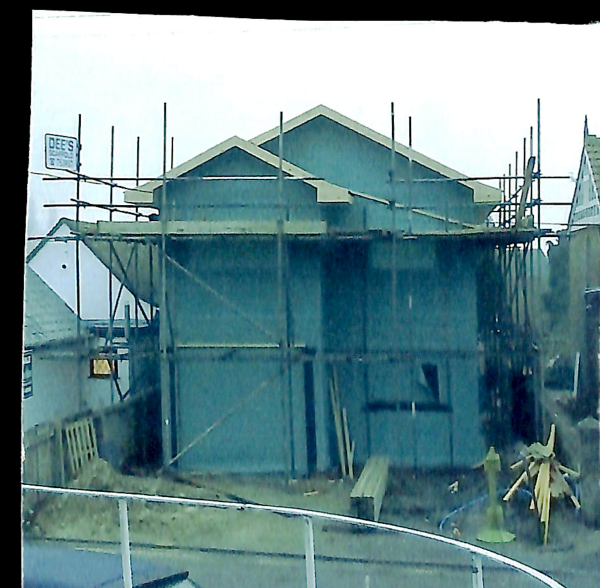
New timber-frame house under construction on site of the old Arnold's coal yard 2002
